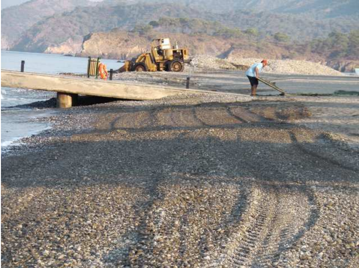
Fig. 9: Excavation work on the beach of the Majesty Club Tuana (Photo: P. Steiner) Abb. 9: Bauarbeiten am Strand vor dem Hotel "Tuana"
